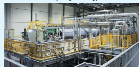
One of the largest water electrolyzers in the world at the Fukushima Hydrogen Energy Research Field
